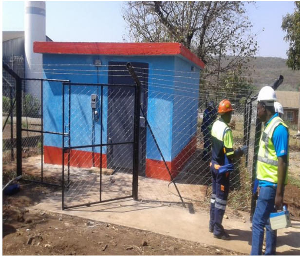
Fig D3: Storage units within facilities with sources awaiting repatriation
