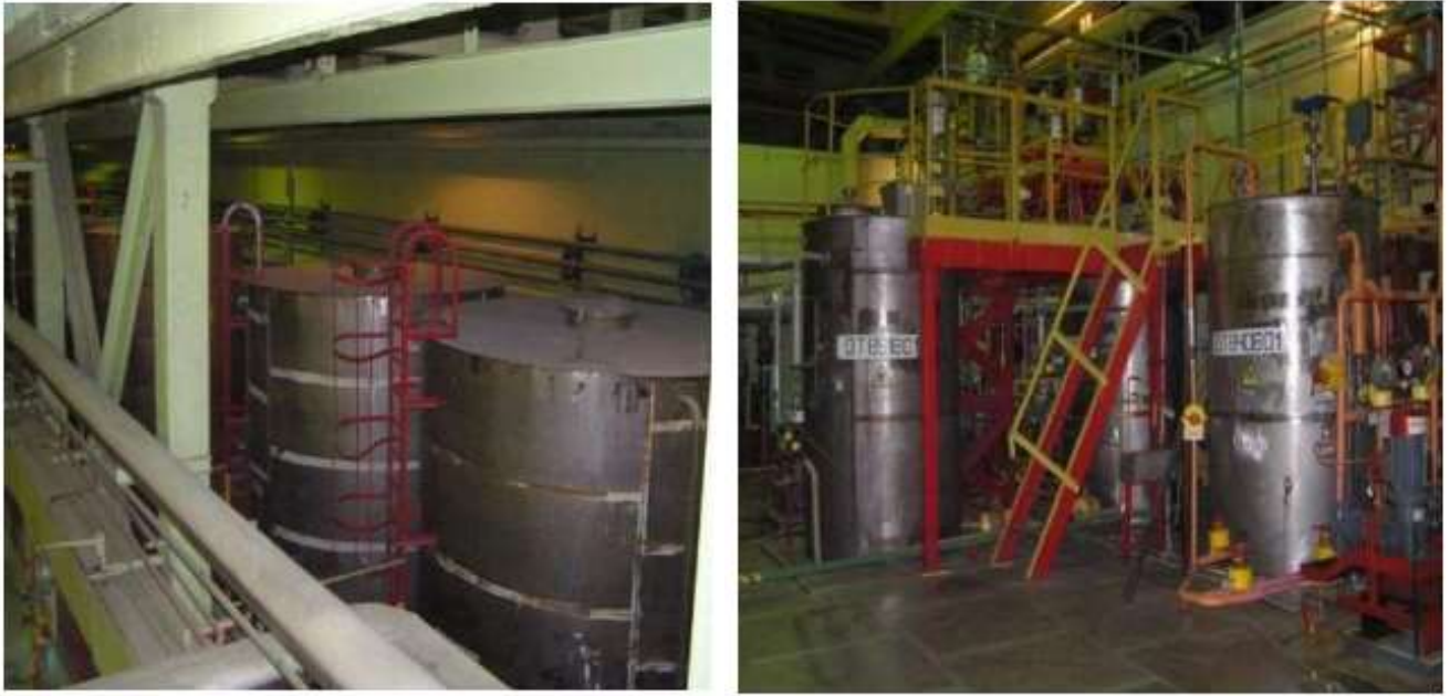
Figure 5. On-site Storage of Liquid Radwaste at NPPs
