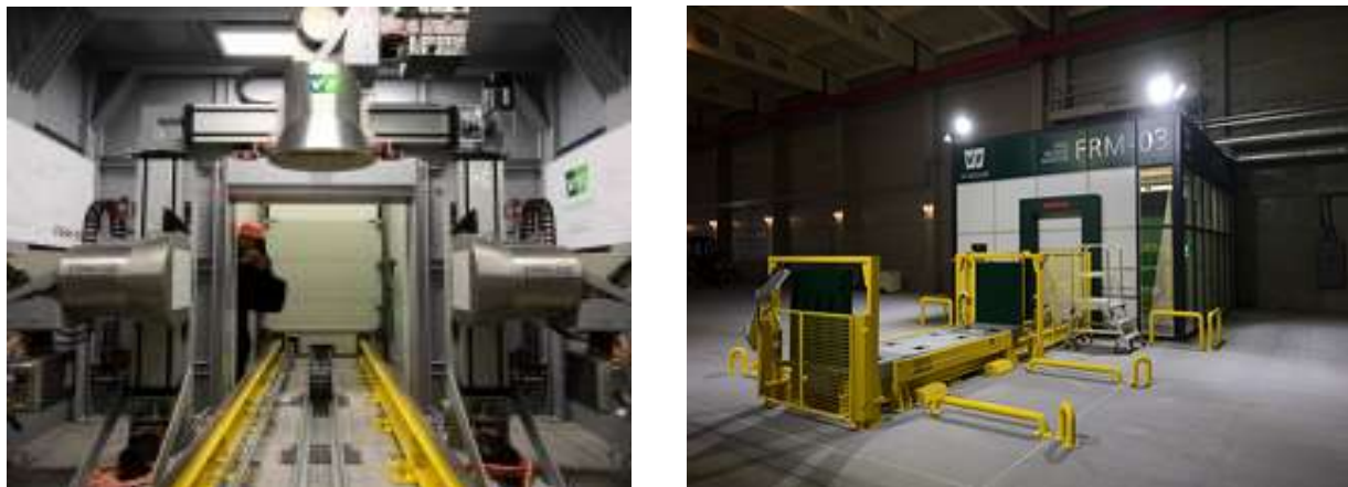
Figure 11. Facility for Release of Materials from Regulatory Control
