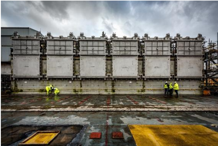
Figure 42: Penetrations into each PFCS compartment, each sealed with a steel door
