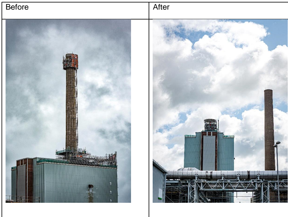
Figure 44: Height reduction of the first generation reprocessing stack
