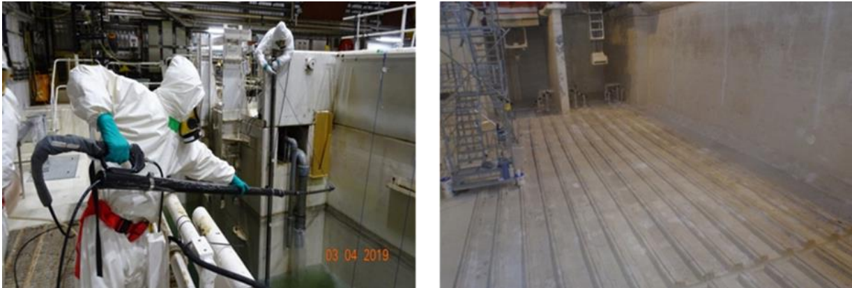
Figure 52: Use of pressure washing from a walkway (left). Fully drained pond (right).
