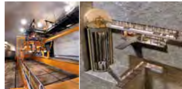
Figure A9 Photo from the top of the silo in SFR and an illustration of the design. Waste packages are placed in shafts in the silo.
