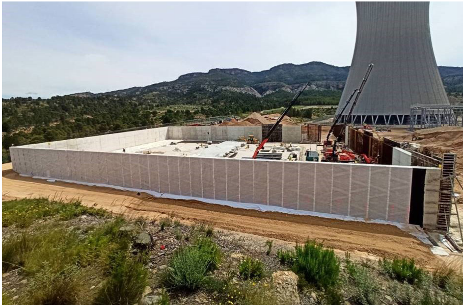
View of the Cofrentes Nuclear Power Plant ITS, now at the licensing stage.
