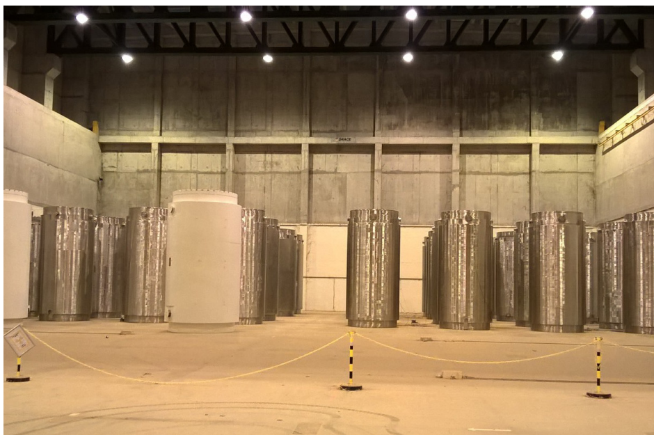
Image of the interior of the Trillo Nuclear Power Plant ITS.
