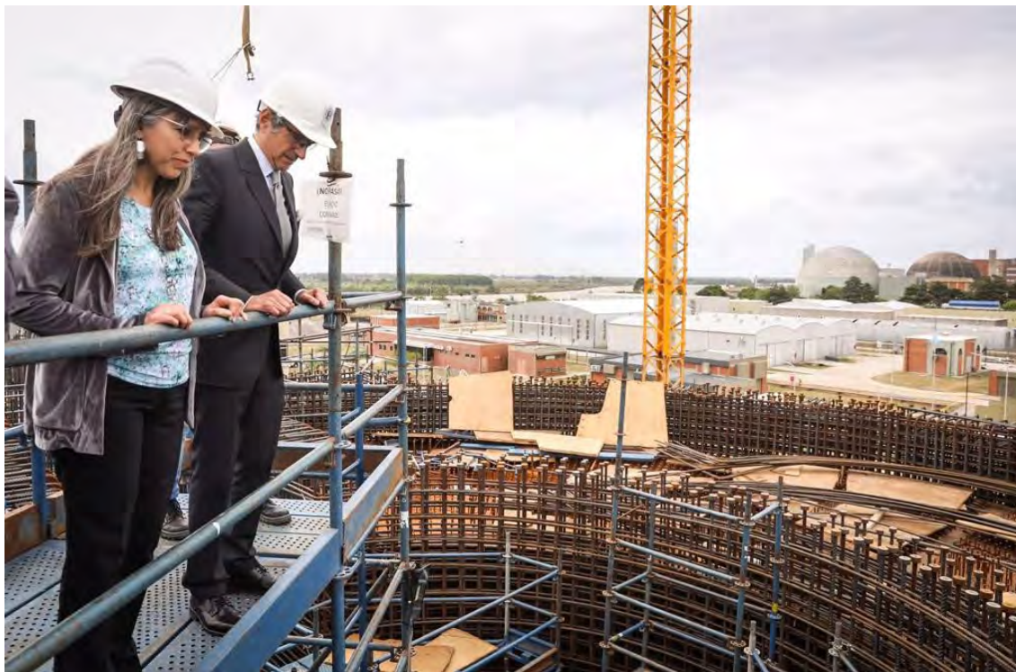
The Director General visits CAREM-25, Argentina's first prototype small modular reactor, currently under construction, October 2022. (Photograph courtesy of I. Dambrauskas/CAREM)
