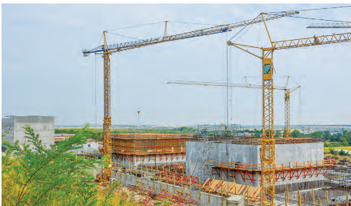
Participants in the DISPONET meeting visited the national repository under construction at the Radiana site, Bulgaria.
