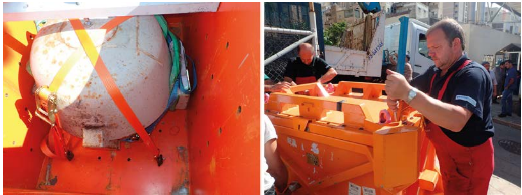
FIG. 2. Preparing for removal of a Category 1 disused sealed radioactive source from Lebanon.
