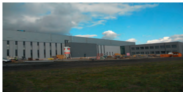
FIG. 3. View of the construction activities for the Nuclear Material Laboratory in Seibersdorf, Austria, November 2012.
