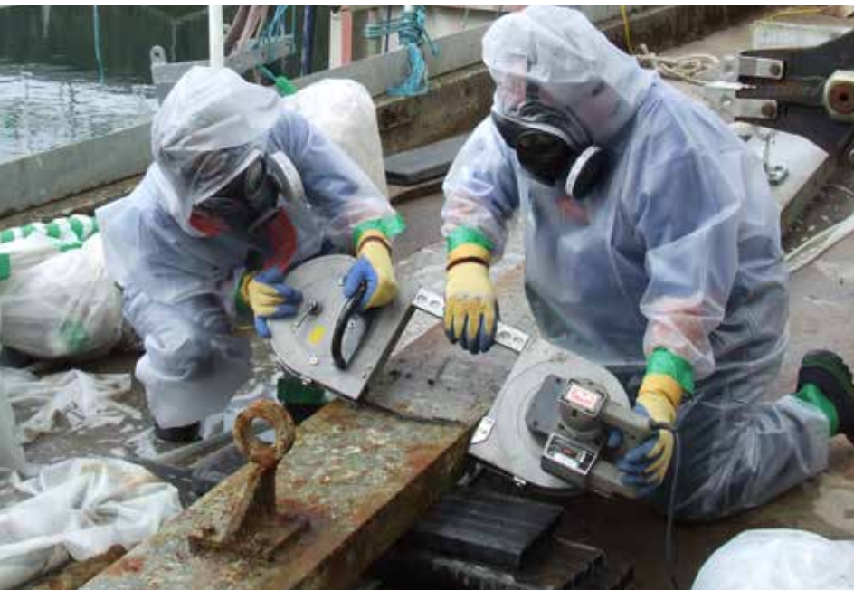
Decommissioning staff cutting down a piece of large metal equipment at a nuclear facility.
