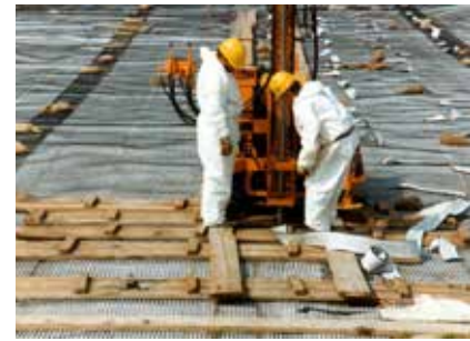
Application of a combined scheme for covering and draining uranium mill tailings.
