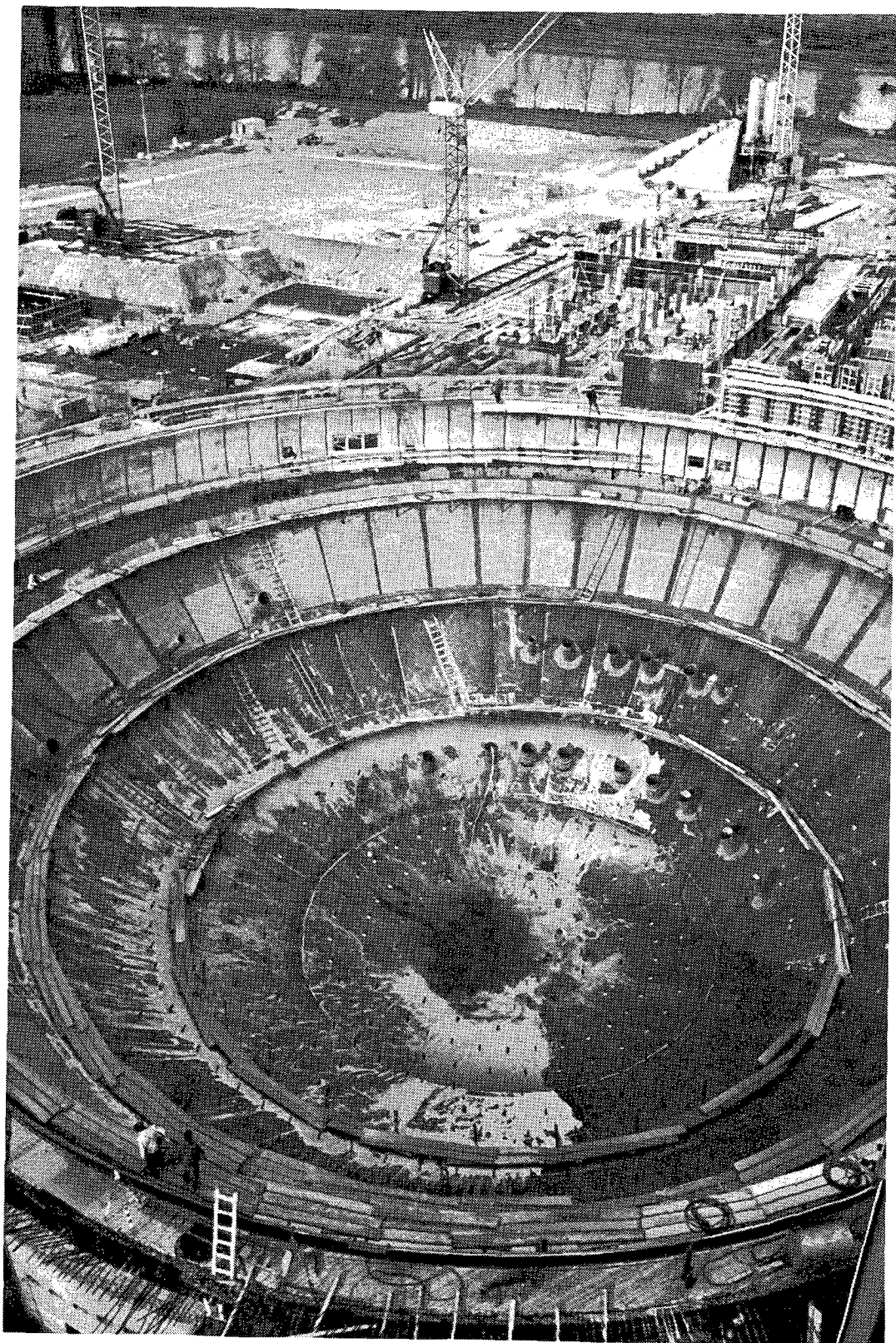
This building site near Biblis on the Rhine bank looks like a huge amphitheatre. It is part of Europe's largest nuclear power plant.
