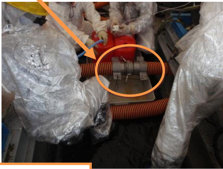
Pipe joint with water leakage
