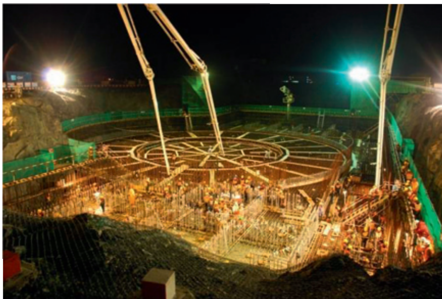
FIG. 1. Pouring the first concrete at the Sanmen nuclear power project site in China.
