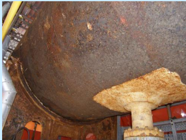
Figure 20 – CO 2 tank 21 as found
