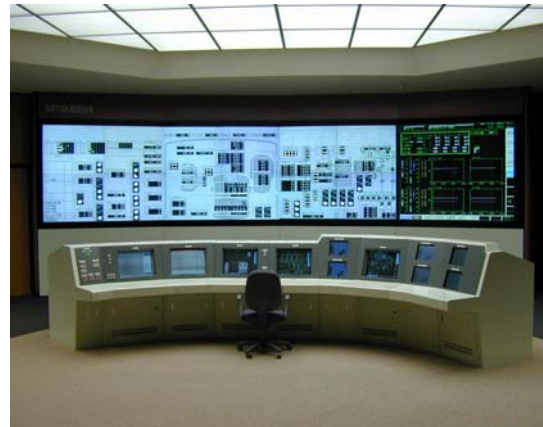
Fig. 12-2 Main Control Panel of Latest PWR (proto type)
