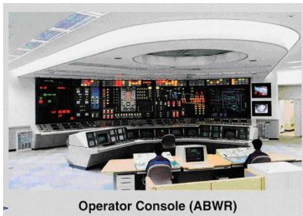
Fig. 12-1 Main Control Panel of ABWR
