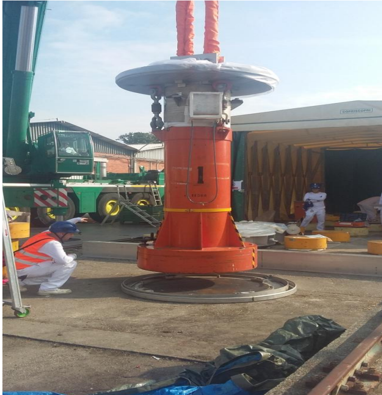
Figure 3: Cold test for the transfer of spent fuel pots from dry-well pits to the dry storage in ESSOR reactor hot cell
