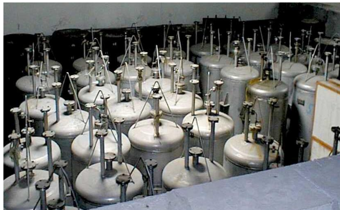
Figure 5: TRINO NPP – Resins from past operation stored in the site
