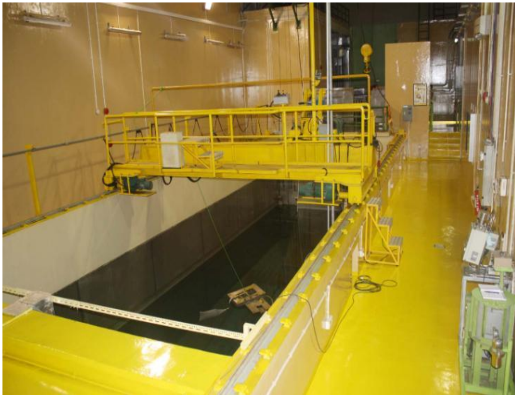
Figure 10. Interim Storage for Spent Fuel Facility
