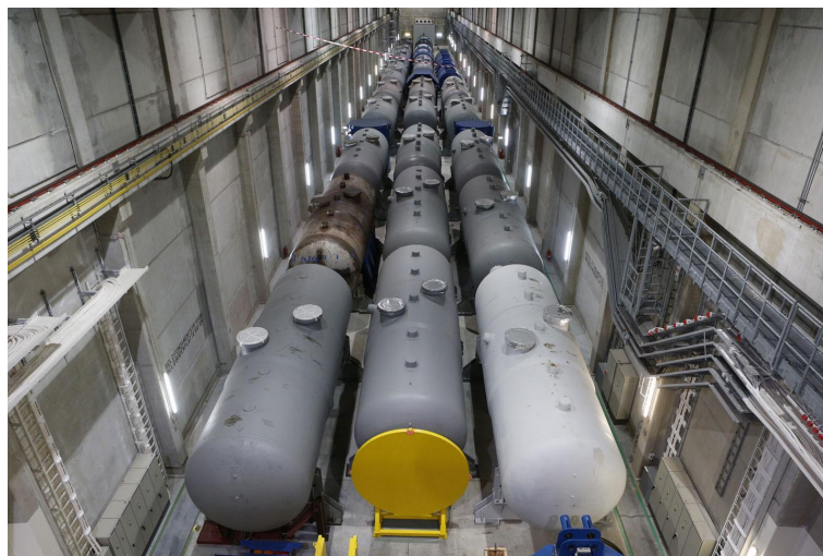
Figure D-7: Decay storage of large components (steam generator) at the Storage Facility North (Copyright: EWN)
