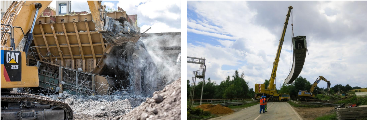
Fig. 2: Dismantling and demolition of the Pipe Conveyer at the Crossen site (2017/2018, copyright: Wismut Archives).
