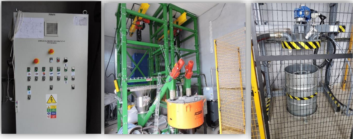
Fig.22 Technological devices of the cementation facility
