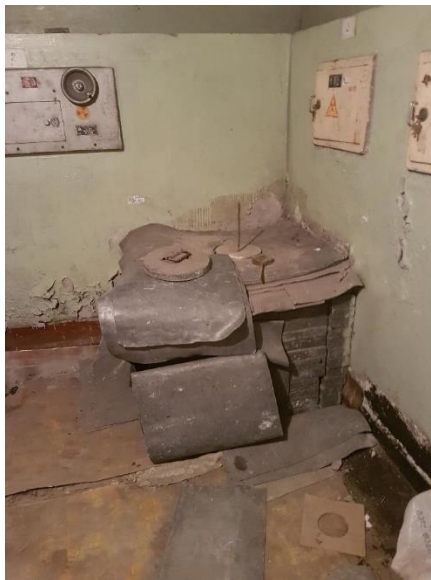
Fig 41 Housing for RaBe source in the corner of the storage room
