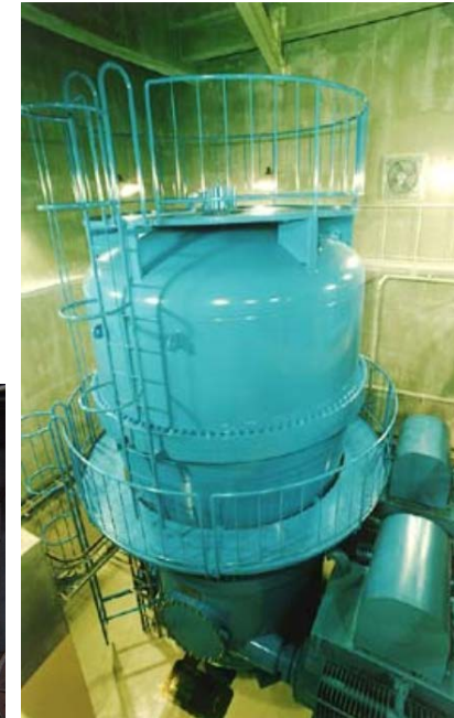
Electron beam (accelerator) irradiation plant
