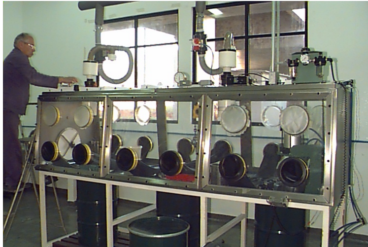
Fig. H.1. Lightning rods dismantling glove-box
