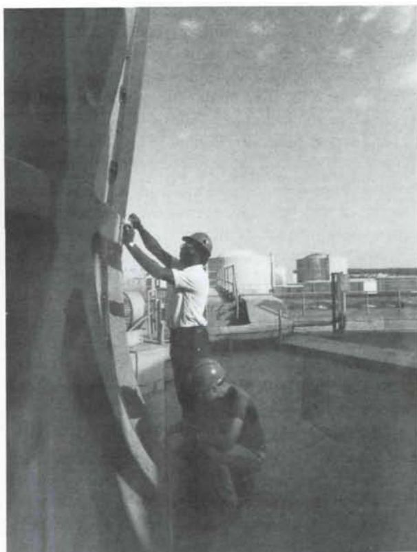
Catawba nuclear plant, USA.
