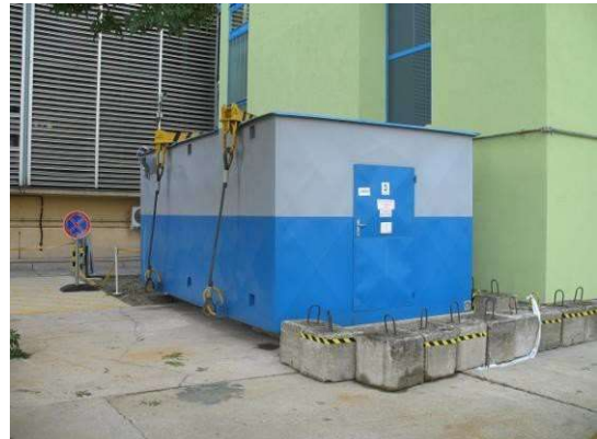
Container battery plant
