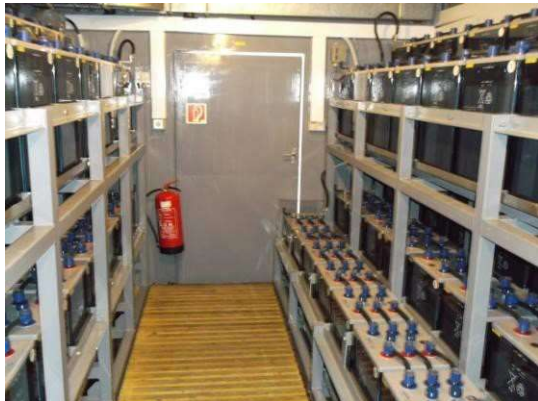
The interior of the battery plant
