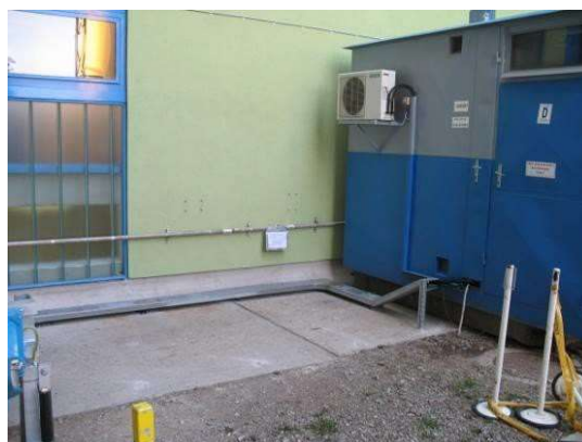
The temporary cable
