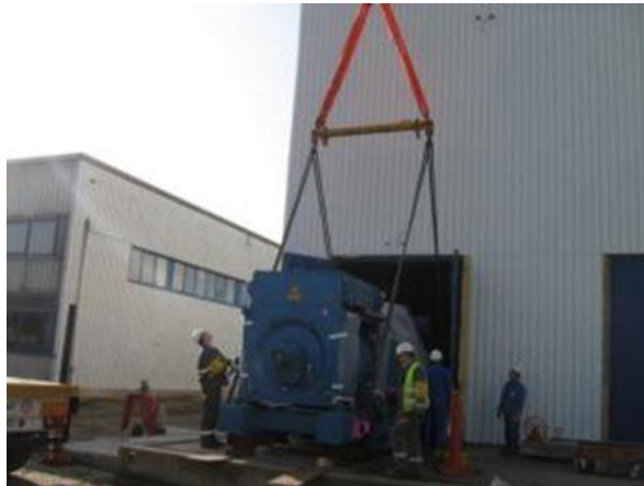
Figure 24 : Installation of new safety diesel generators in the DGG of units Doel 1 & 2
