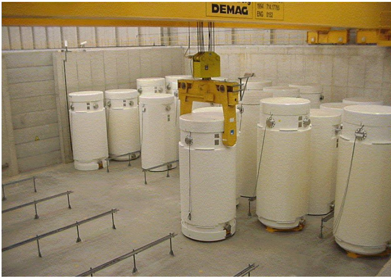
Figure 30 : Intermediate Storage Building for Spent Fuel of Doel
