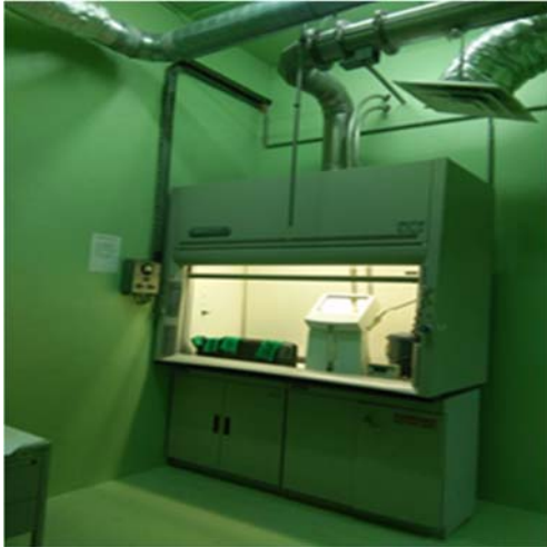
Pneumatic Transfer System (PTS) terminal
