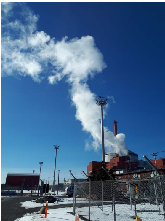
FIGURE 23. Commissioning tests of main steam relief trains at Olkiluoto 3. Source: STUK.
