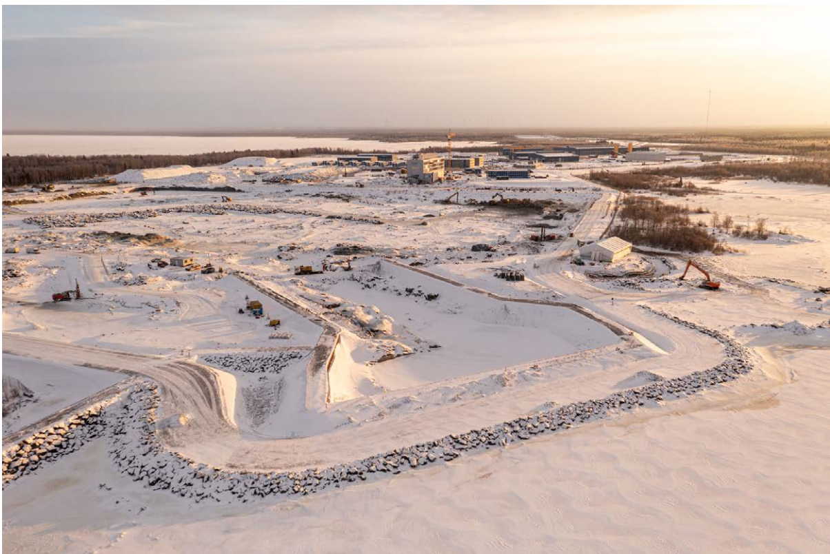
FIGURE 25. Hanhikivi site in Pyhäjoki selected for Fennovoima new NPP, cooling water inlet channel with temporary dam and NPP plant pit excavation (FH-1, February 2022). Source: Fennovoima.
