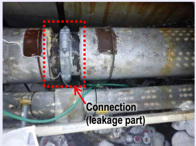
<Leakage part of the connection after moving insulator> * Refrigerant (brine): Liquid calcium chloride (the same ingredients as the snow melting agent sprayed on roads during snow fall)
