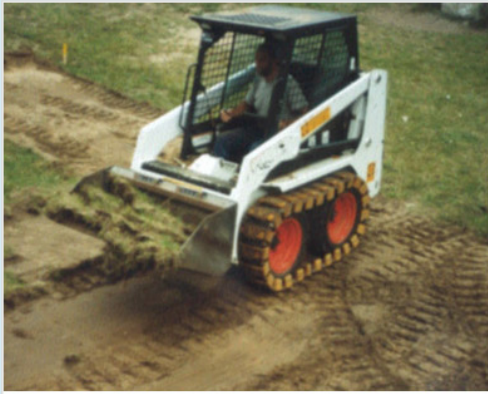
Figure 3. Removal of contaminated topsoil with a 'Bobcat' mini-bulldozer in the Bryansk region in 1997 (Courtesy of Risø - DTU National Laboratory Roskilde, Denmark)
