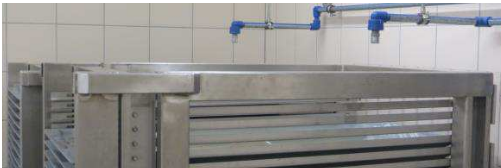
Figure 19. Overflow system. Two pipelines placed over the steel rack to fill the trays with water using the overflow system.
