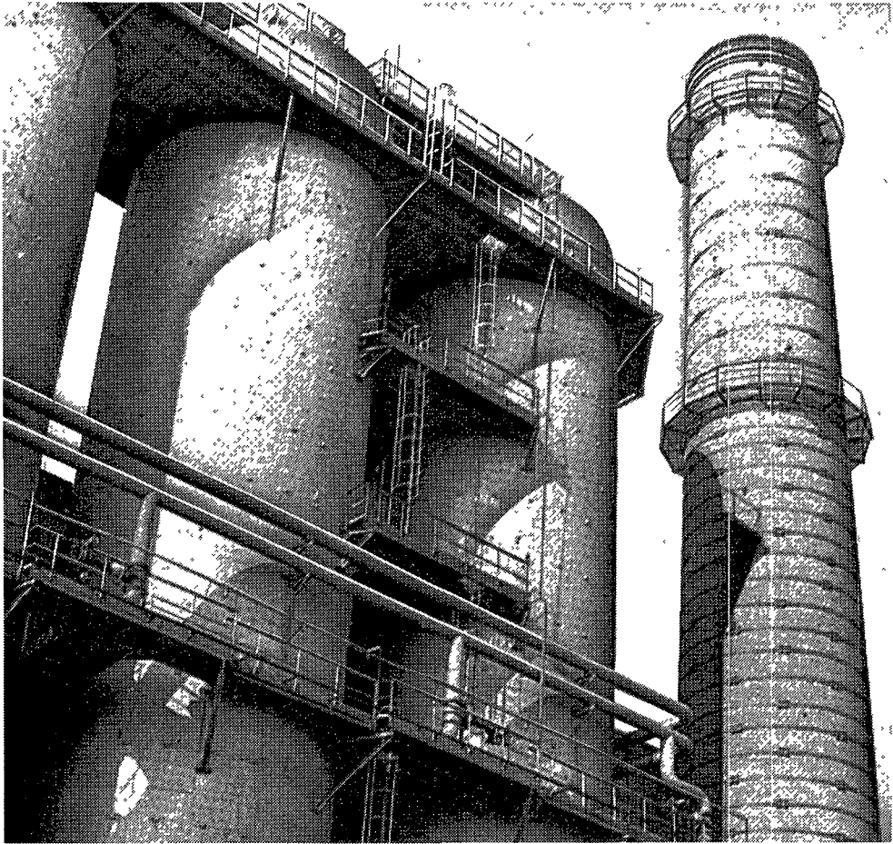
Air preheater of the U-25 facility at the High Temperature Institute of the USSR Academy of Sciences
