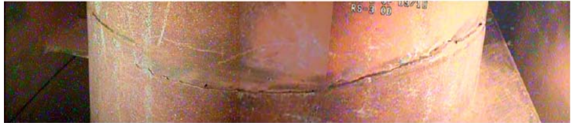
Cracking of riser pipe JP 9/10 during RF-13
