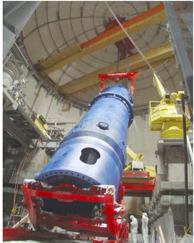
A view of steam generator replacement: steam generator rigging inside a containment
