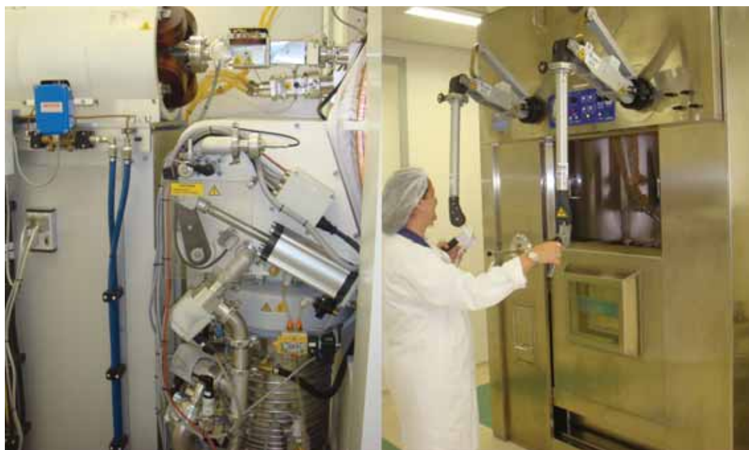
FIG. 2. A cyclotron beam extractor (left) and production hot cell (right) for manufacturing PET radionuclides in Recife, Brazil.
