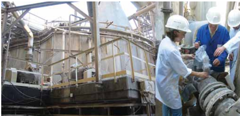
FIG. 3. Optimizing phosphoric acid production using radiotracer techniques at a plant in Tunisia.
