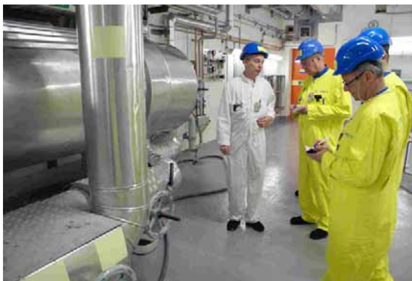
FIG. 1. OSART members inspecting equipment at the Forsmark nuclear power plant in Sweden.
