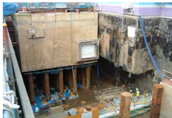
FIG. 2. Removal, cleaning and replacement of oil contaminated soil below the pile foundation of a non-safety related structure at the Kashiwazaki-Kariwa nuclear power plant.
