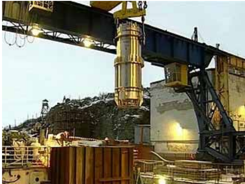
FIG. 3. Removal of submarine spent nuclear fuel from the former naval base at Gremikha for reprocessing at the Mayak plant in the Russian Federation.
