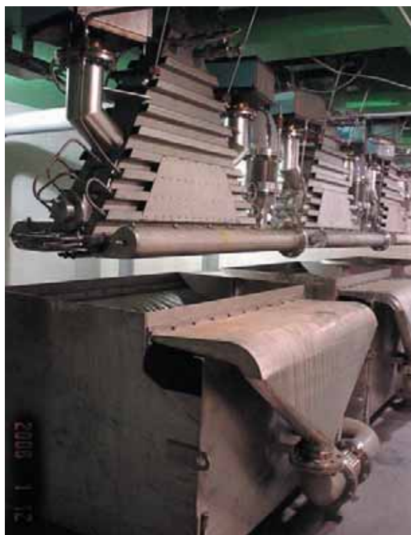
FIG. 1. The first industrial scale electron beam wastewater treatment plant in operation in the Republic of Korea.
