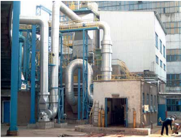
FIG. 1. Pilot plant for electron beam flue gas treatment at the Maritsa East 2 thermal power plant in Bulgaria.
