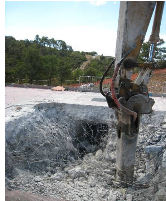
Harmonie reactor, CEA
