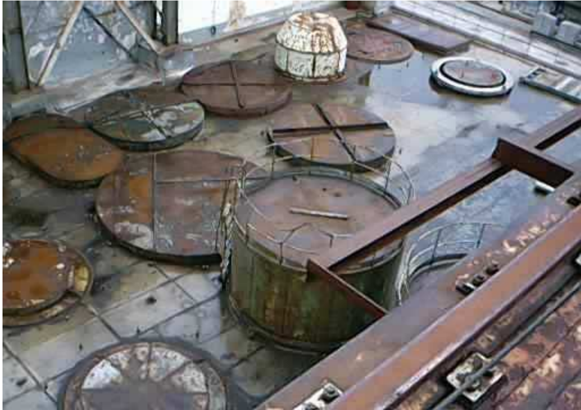
Photo 3. Process hatch covers
