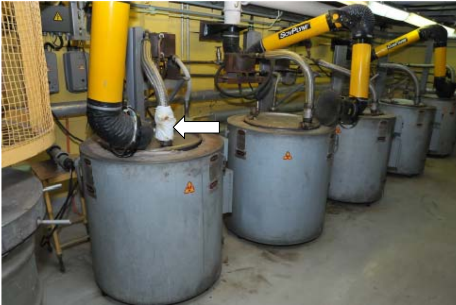
Figure 2. Ad-hoc repairs carried out at a radioactive waste management facility.
