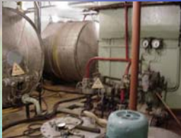
tank facility of the covered slipway dock for the LRW collection and temporary storage;
