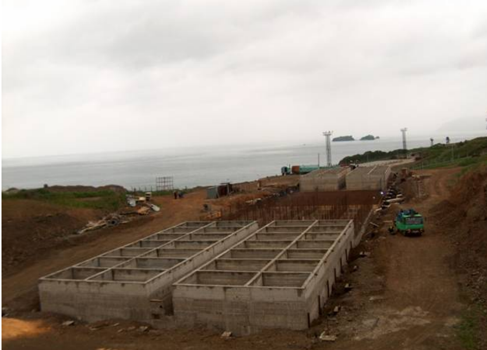
Figure 8. Construction of the solid RW storage at the DalRAO site in the Sysoeva Bay
