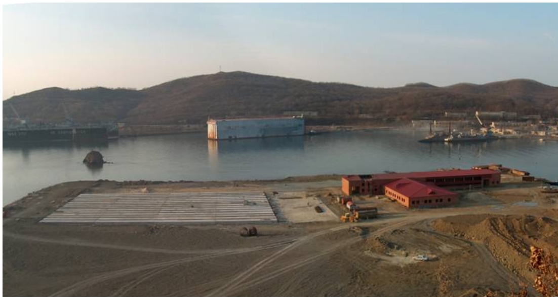
Figure 6. Construction of the coastal RC storage facility in the Razboynik Bay at the Far East
