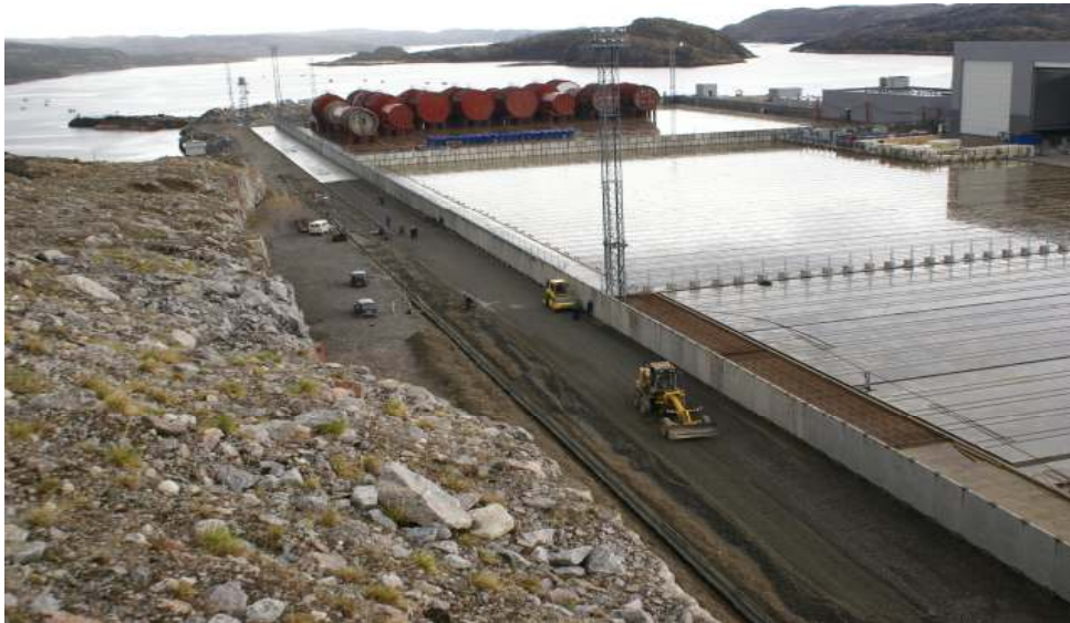
Long Term Storage Facility Reactor of Compartments funded by Germany
