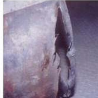
FAC on Ø14" heater drain extraction line to high pressure heater (HPH) at Arkansas unit 2 (USA, 1986)
