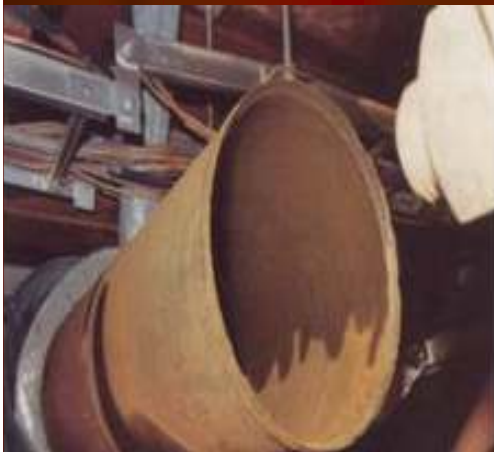
FAC on Ø9" elbow of HPH drain line at Millstone unit 2 (USA, 1991)
