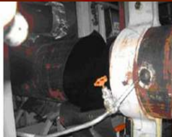
Wall thickness reduction from 10 to 1.5 mm on feedwater piping at Mihama unit 3, 2004
