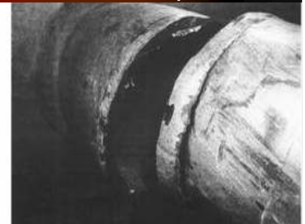
Wall thickness reduction from 8 to 1.5 mm on feedwater bypass at Balakovo unit 2, 2004
