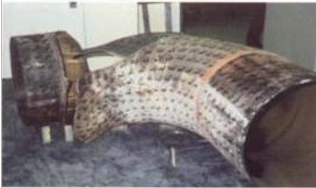
Ø18" elbow wall thickness decreased from 12.7 to 1.5 mm on feedwater pump inlet at Surry, 1986
