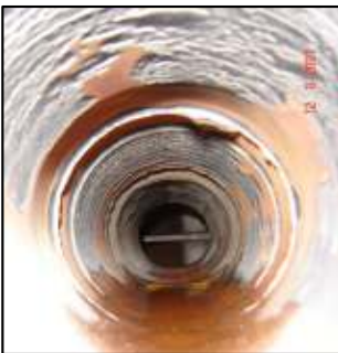
surface degradation of base material
