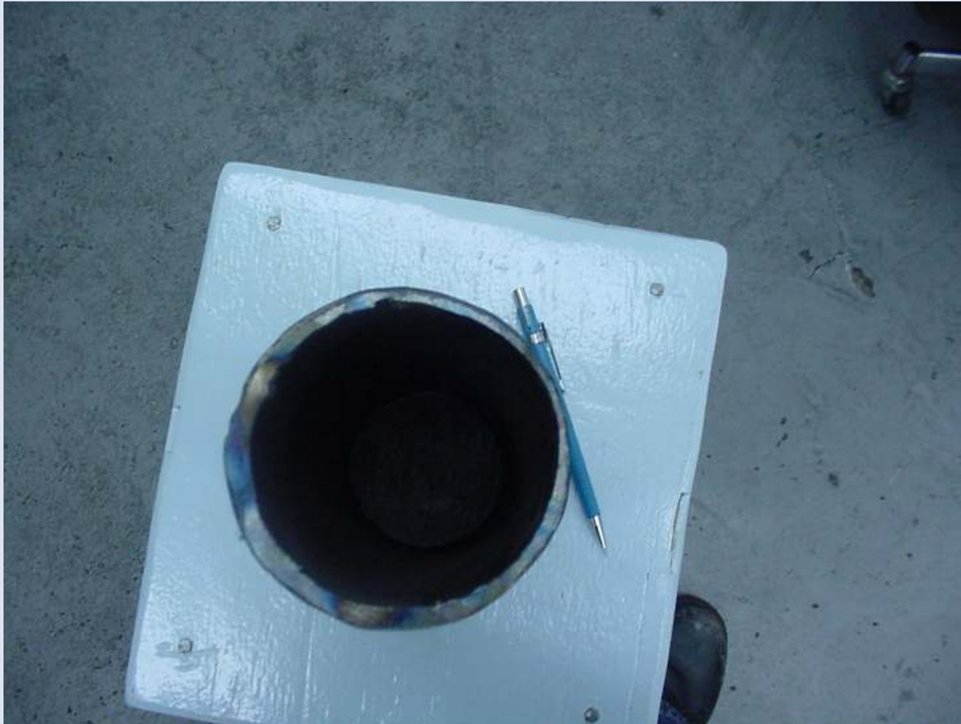
Heater Drain Line – DN 3”
