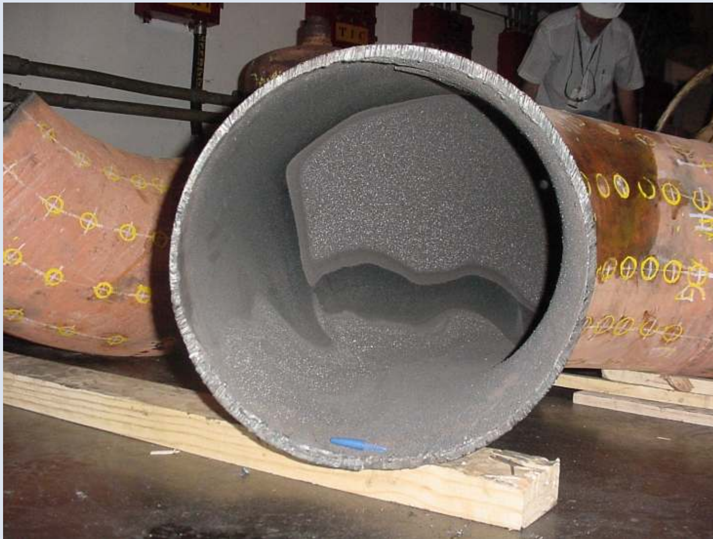
Steam Extraction Line – DN 16”
