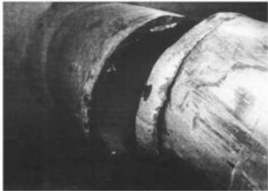
Russia, Balakovo NPP, 11.2004, unit 2, 1000 MW
