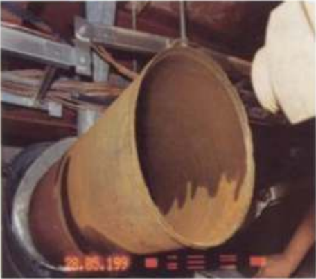
Main Feedwater Pipeline
